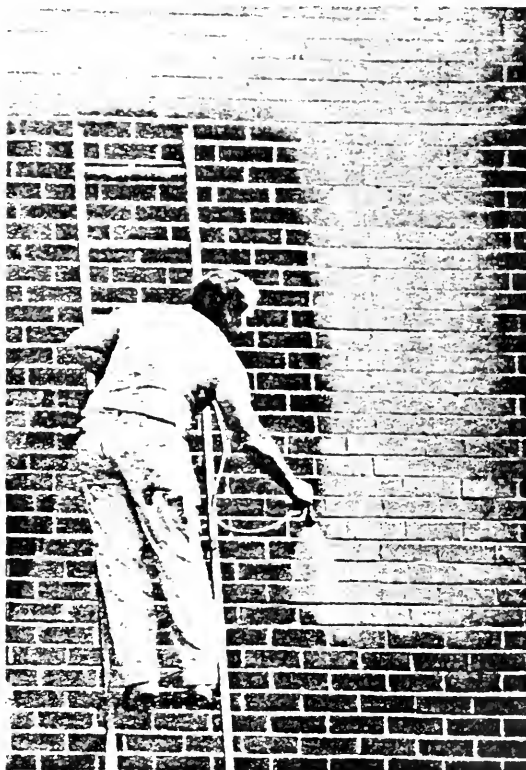
A construction worker at the Villages of Montpelier, formerly known as the Pumpkin Hill-South Laurel Apartments, sprays paint—not graffiti—on the brick wall of one of the buildings undergoing a complete overhaul at the complex east of the Baltimore-Washington Parkway and south of Route 197.
